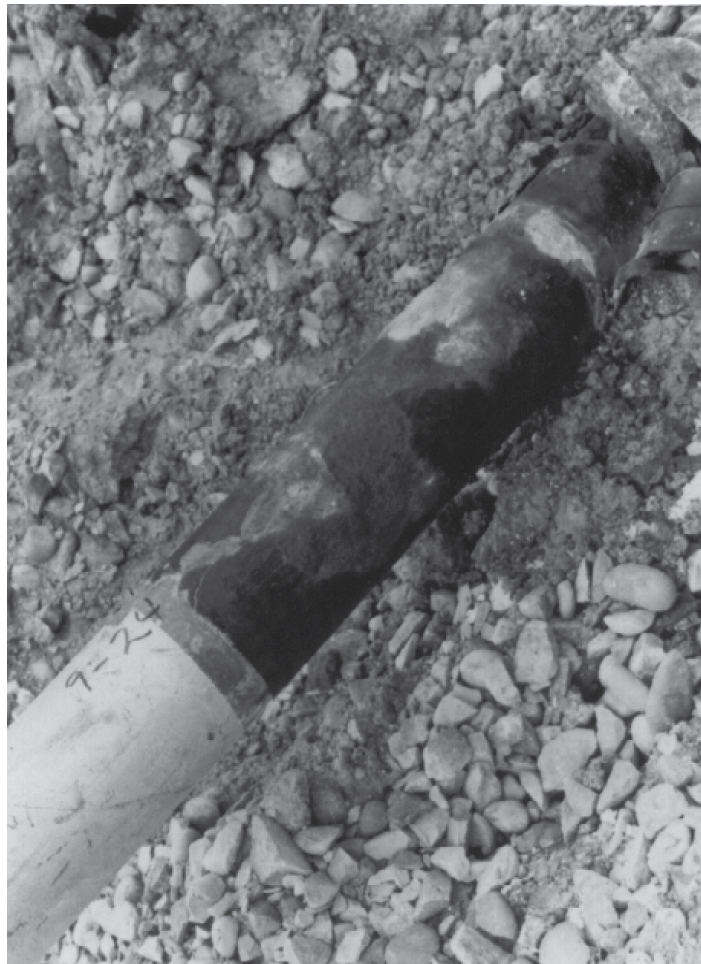
Figure 23—Underground Piping Corrosion beneath Poorly Applied Tape Wrap
