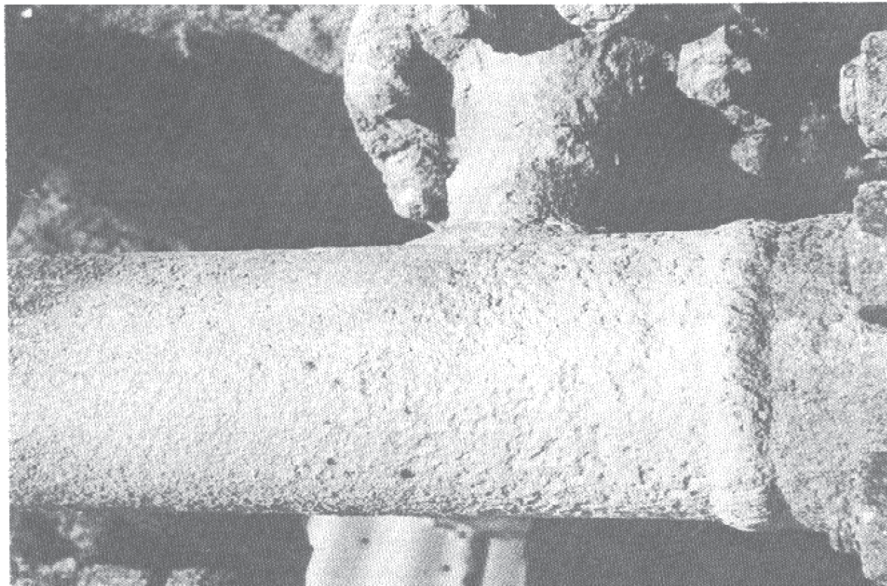
Figure 20—Severe Atmospheric Corrosion of Piping
